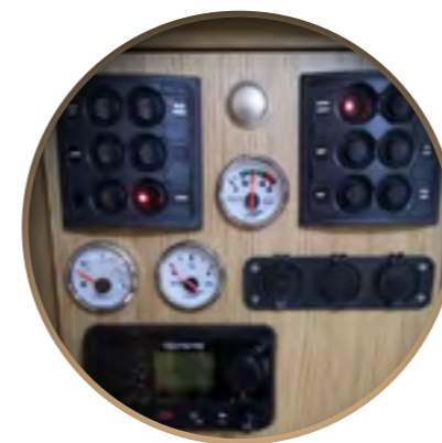
Standard BEP panels with WEMA gauges.
